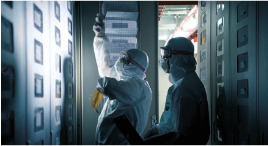
Taking stringent measures to protect our field engineers by putting on Personal Protective Equipment (PPE) when installing services at quarantine centres
